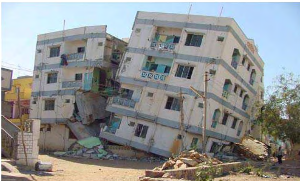
(b) Collapse of ground storey RC columns (soft storey) during 2001 Bhuj Earthquake
