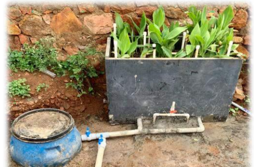
Tertiary Treatment (Constructed Wetland)
