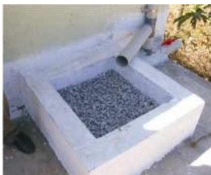
Sand bed filter over a rainwater storage tank
