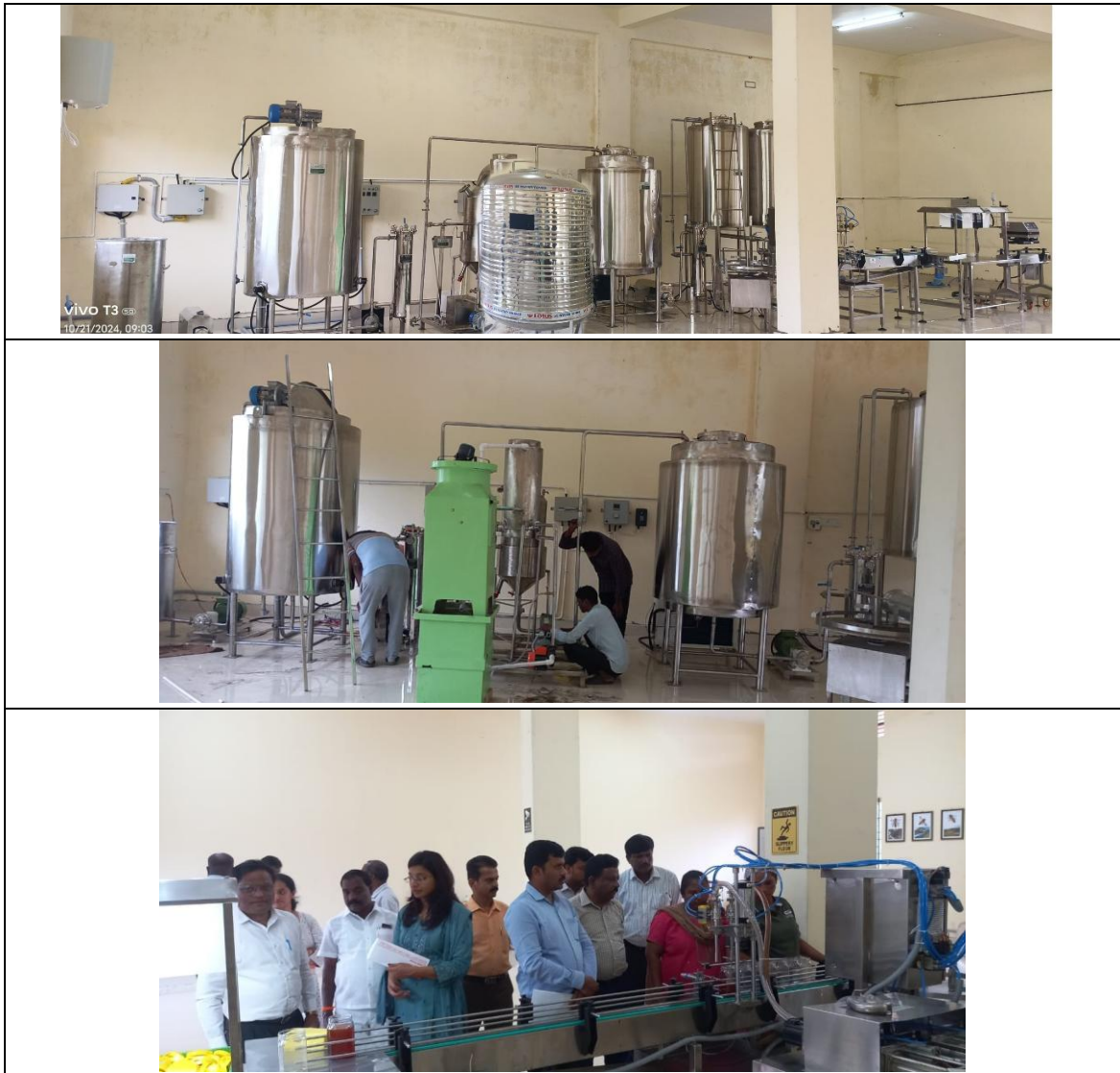
Honey processing and bottling plant at Karnataka State LAMPS Cooperative Federation building, Hebbal Industrial Area, Mysuru.
